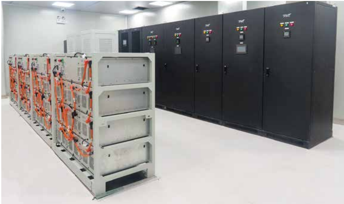
The Integration of IDC Backup Power
