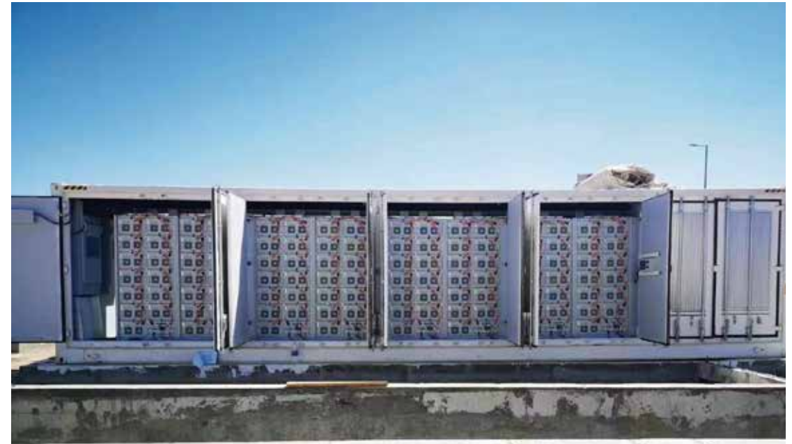
Photovoltaic supporting facilities
