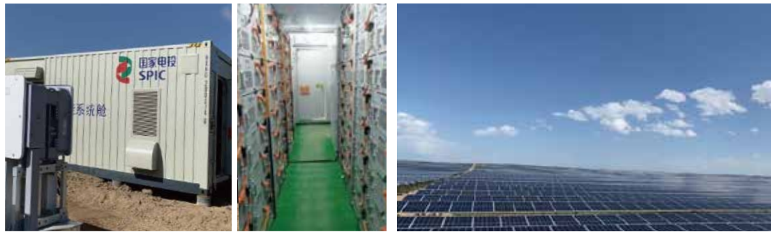
Utility ESS · Power generation side
