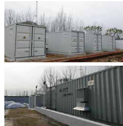
Utility ESS · Transmission & Distribution side
