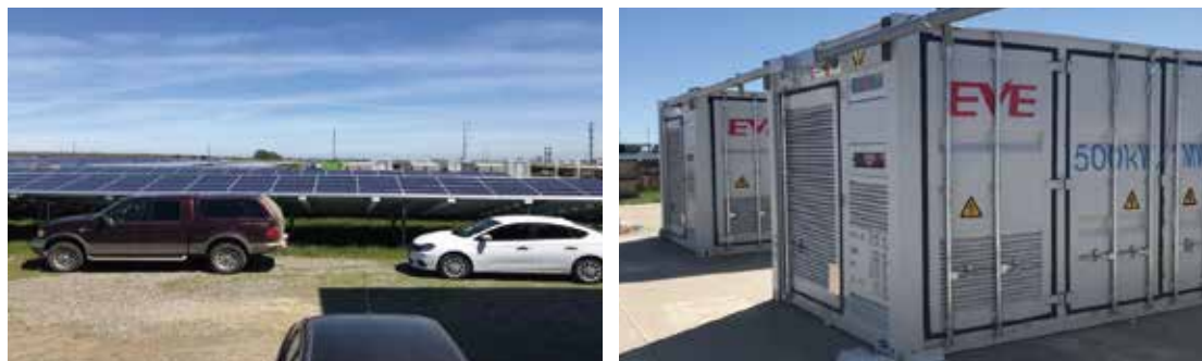
Utility ESS · Power generation side
